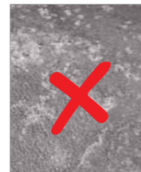
Standard coating: Corrosion
